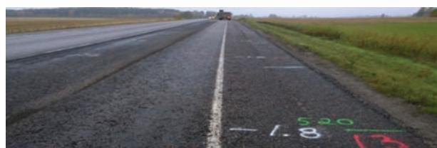
Figure 9. 3-D guiding machine control notes painted in surface of road (green = position in length of road (m);
