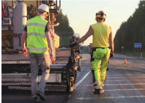
Figure 6. Paving machine operator in work with 3-D guiding machine control system (Roadscanners Oy).
