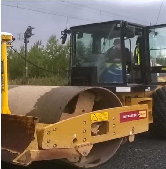
Figure 4. The Trimble machine control system was used in soil compactor for quality measurements.
