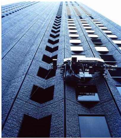
Figure 6. Single Task Construction Robot applied by the company Taisei to automatically coat and paint the façade of a high-rise building
