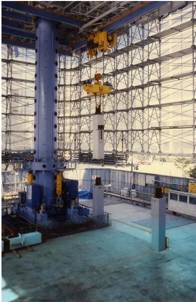
Figure 4. The concept of Robot Oriented Design applied in an automated construction site (SMART) of the company Shimizu.
