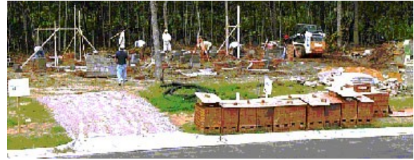
a) Labor is Establishing Foundation Walls, Brick is Staged at Road, Bobcat is Operating
