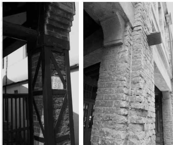
Figure 4. mixed of materials used on the historic building on different stages of renovation, steel frames were used to support the structure
