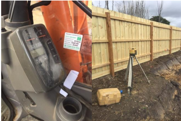
Figure 5. Excavator in Stationary Position; Cabin with LCD Control Panel; TopCon Laser Transmitter
