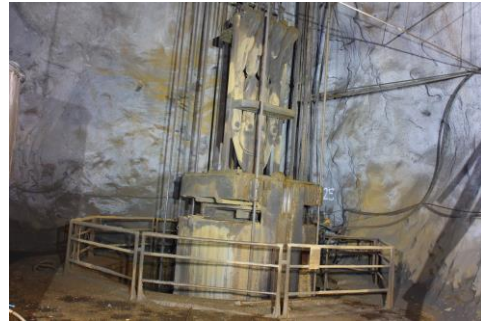
Figure 3. Overall image of the measurement position in relation to the upper part of the elevator.
