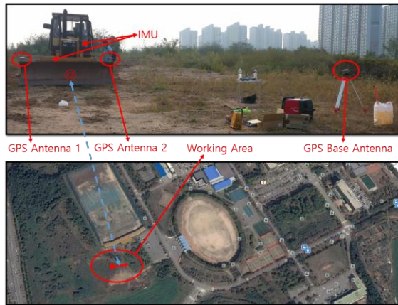
Figure 5. Experimental setup: Dozer, sensors and location that is Hanyang Univ. at Ansan
