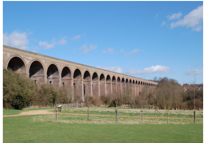
Figure 2: The Chapel viaduct, Essex, United Kingdom, a masonry structure many visible damages.
