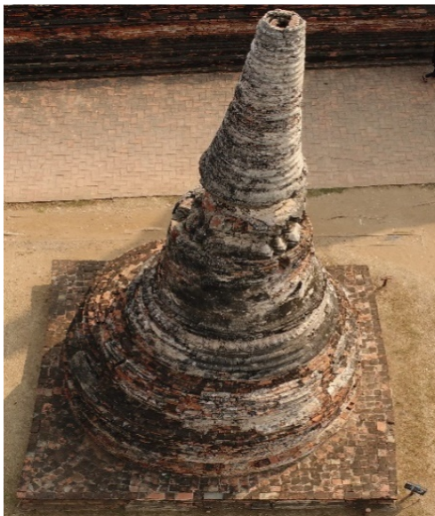
Figure 1: A masonry structure from Ayutthaya, Thailand, which is inaccessible for manual inspection. Hence, images are acquired using a drone.
