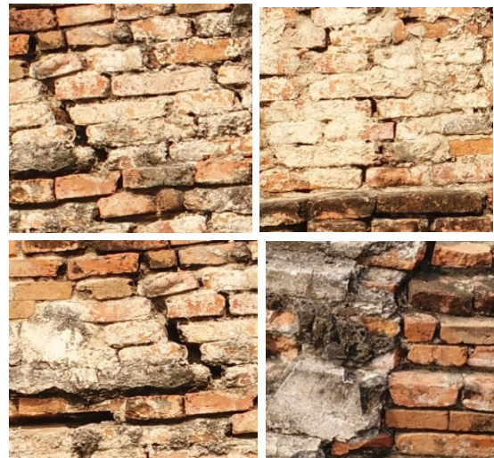
Figure 3 :Sample images of cracks in masonry structures
