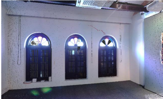
Figure 7. Point clouds of scan19 with cracks
