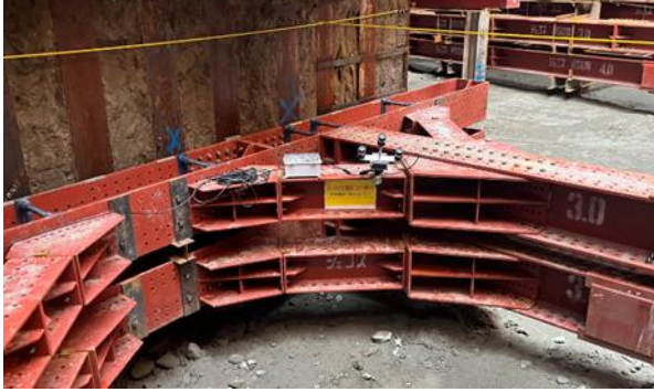
Figure 4. LiDAR installation in Section 1
