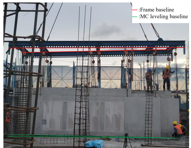
Figure 1. Rough chain adjustment by workers leads to module tilting and extra structural bending.
