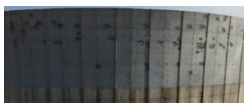
Figure 5. Captured image of spalling near the top ring of an aging cooling tower.
