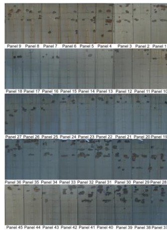
Figure 10. The projected top ring panels of defects.
