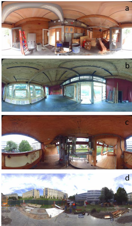
Figure 3. Point clouds captured at different times during the project: (a) before deconstruction, (b) after removing furniture and exterior walls, (c) after removing door and window frames, (d) after lifting the roof
