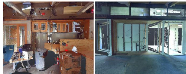
Figure 7. Metal studs behind the kitchen region are invisible in Scan 1 (left) but become visible in Scan 2 (right)
