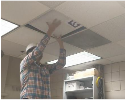
Figure 1. The construction process involves repetitive tasks with different objects, such as ceiling tile installation, the tiles are maneuvered and placed repetitively at different locations.
