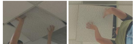
Figure 3. Example of the ceiling tile installation demonstration video with two different camera viewpoints.
