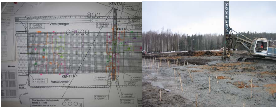
Figure 1. Example of current 2D deep stabilization plan with columns to be stabilized between 1.25 m intervals (left), traditional Piling Process (right): no 3D positioning for the machine, instead wooden target sticks, only 2D drawings available, manual control system for any movements of the machine, quite stable (constant) feeding of stabilization material per point, poor measurement and saving of machine parameters during the work, poor as-built documentation and non-homogenous columns demand cases using special PDA measurement technique.
