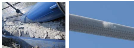
Fig. 1 Ice formation on a stay of Incheon Bridge
