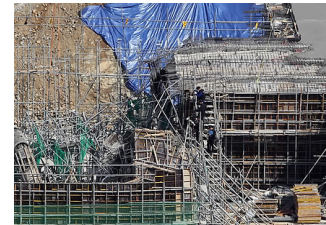
Fig. 1 A case of construction failure
