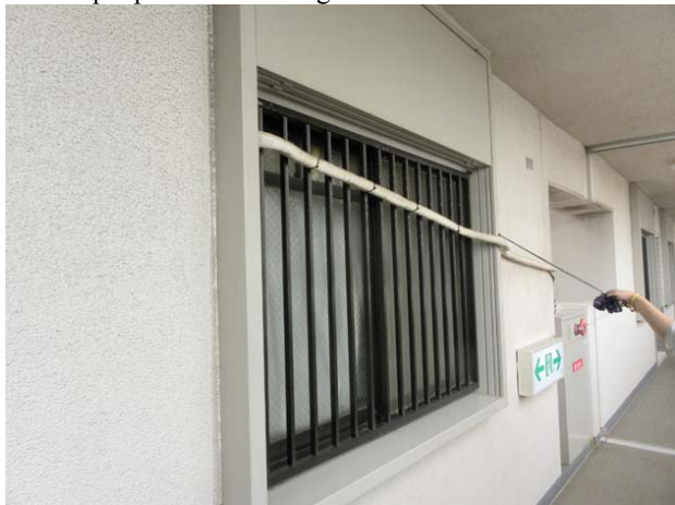
Fig. 7 Obstacle on fire prevention shutter
