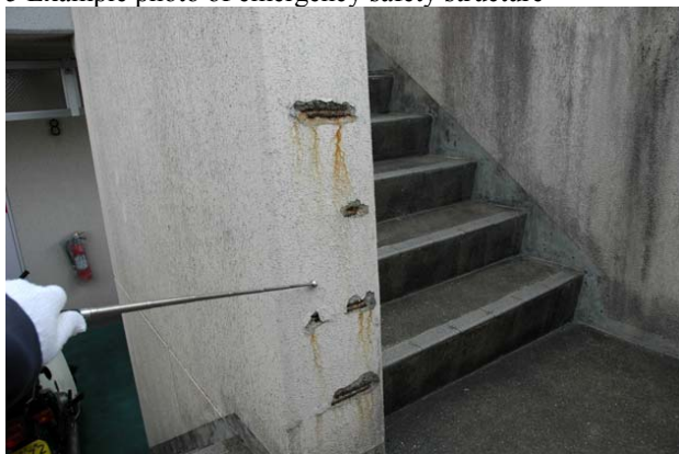
Fig. 8 Rust in the reinforced concrete at outside stairs
