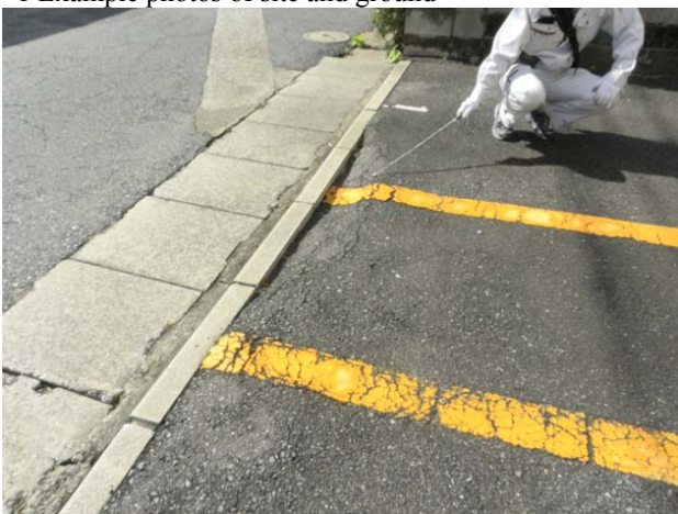
Fig. 4-1 Cave-in on the ground
