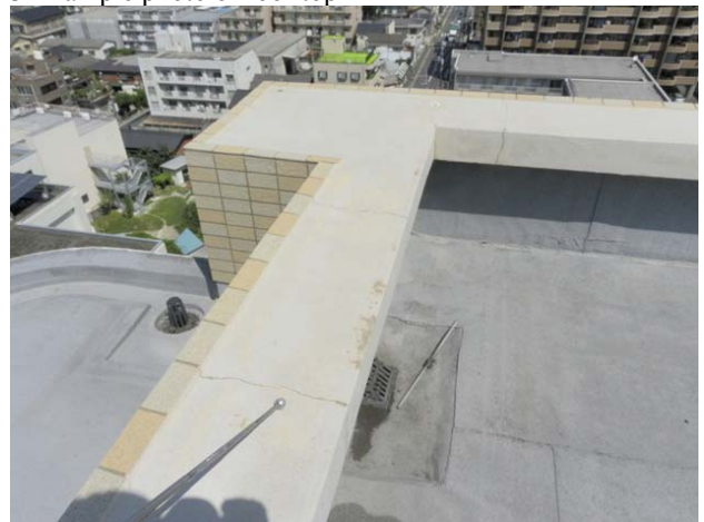
Fig. 6 Crack in the concrete parapetto on the roof top
