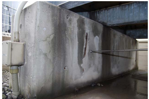
Fig. 4-2 Crack in the concrete base of a water receiving tank
