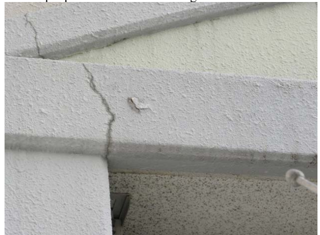
Fig. 5 Crack in the concrete outside wall
