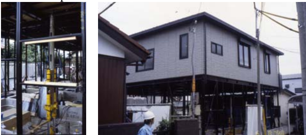
Fig. 3: J-Up System: Hydraulic presses push up the building floor by floor enabling efficient construction on the ground floor level. Sekisui House.
