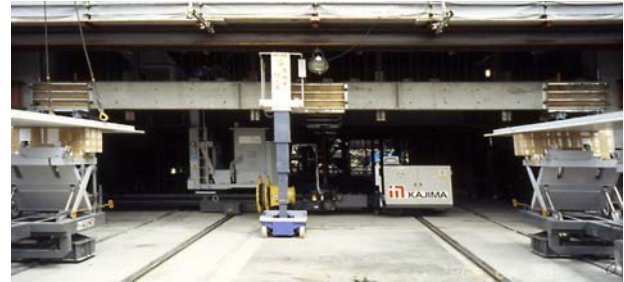
Fig. 6: The AMURAD Construction Strategy: for floor-wise up-pushing of the whole building. Kajima, Japan.
