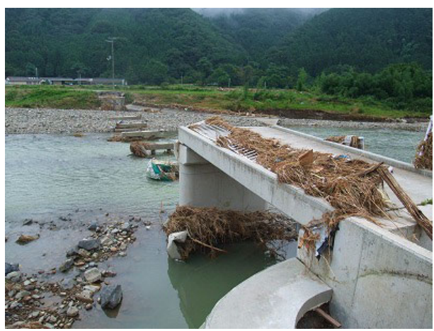
(b) A collapsed pier on the Chigusa River
