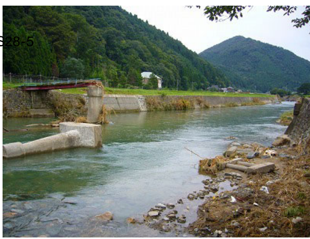
(a) A collapsed bridge on the Ibo River
