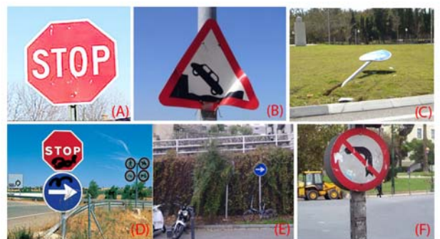
Fig. 2. Different examples of damages in traffic signs: (A) paint deterioration, (B) folded sheet, (C) pole bent, (D) vandalism, (E) concealment by vegetation and (F) adhered substances.
