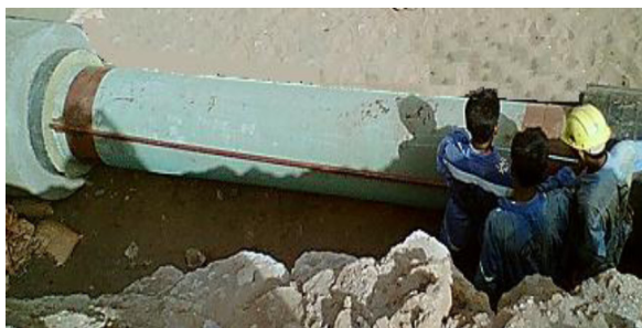
Fig. 2. A typical “tie in” joint between a river crossing and mainline section of a pipeline
