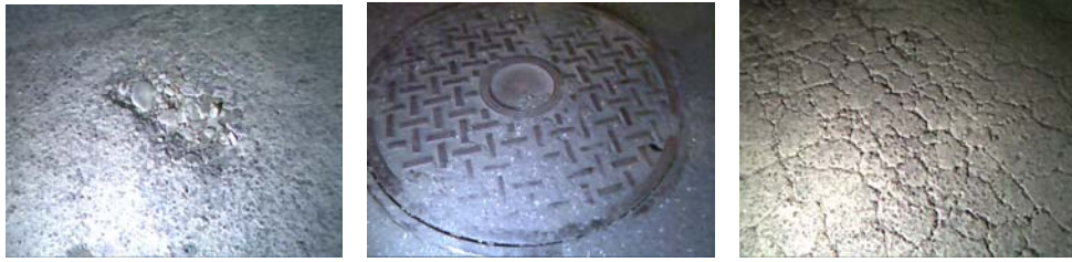
Figure 8: Distress Photographs Taken by P3-AT (Point 1, 4 and 5)
