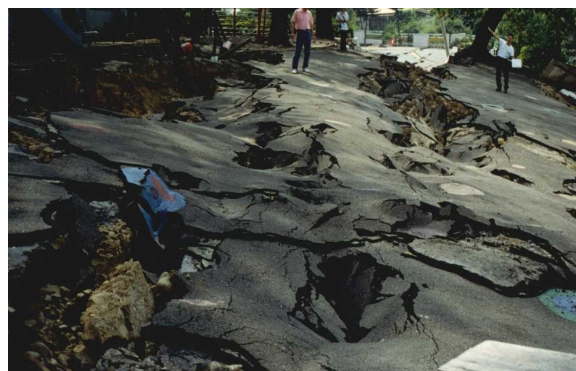
Figure 2 Damages of roads caused by Chi-Chi (921) Earthquake
