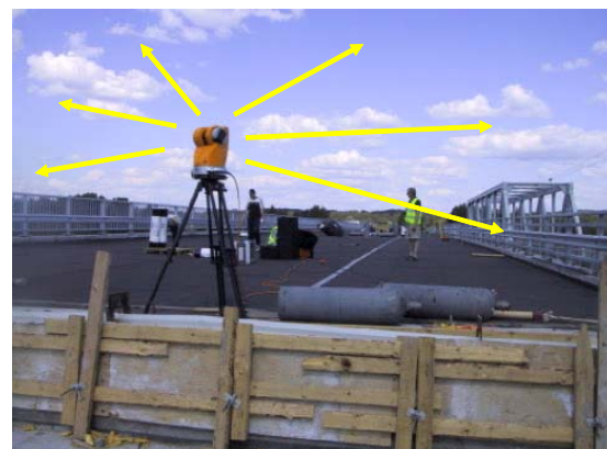
Figure 5. Testing a “dome-like” (Callidus) 3-D laser scanner in the geometric inspection of the concrete deck slab of Pessankoski Bridge.
