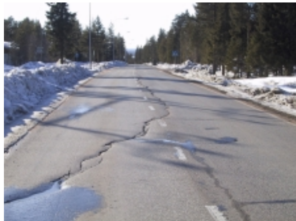
Figure 1. Road rehabilitation process begins with existing road damage – a case in Finland.
