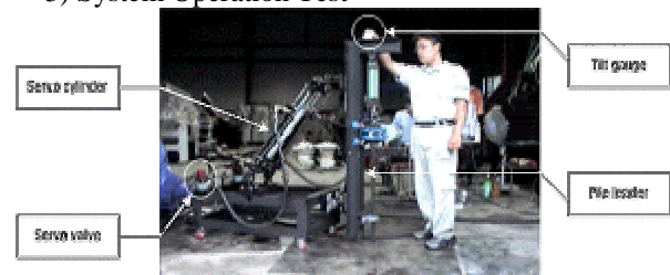
Figure 7. Tilt Gauge & Servo Valve Function Test
