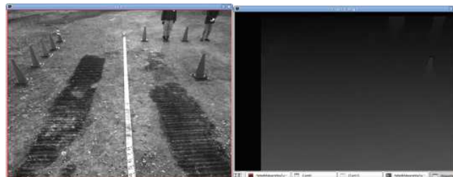
Figure 7 – Excavator: Travelling Backward, Workers: Standing Still at a distance of about 6m and 2m/4m away from the center of the Excavator
