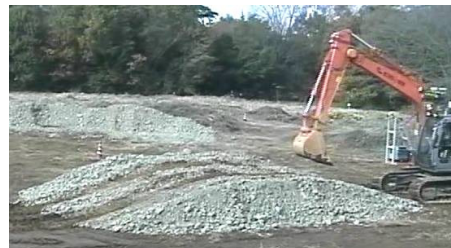
Figure 2 – Obstacle of crusher-run stone after several trials to drive and get over
