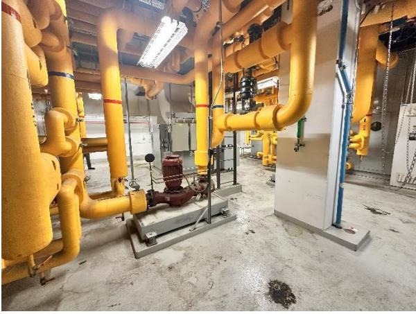
Figure 3 Mechanical Room for the Experiment
