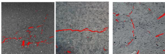
Figure 1. Examples of crack segmentation
