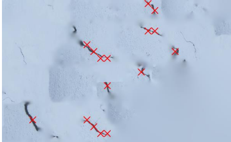
Figure 12. Texture of the wall with cracks identified
