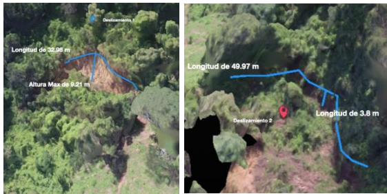
Figure 5. 3D measurement of the Landslides 1 and 2
