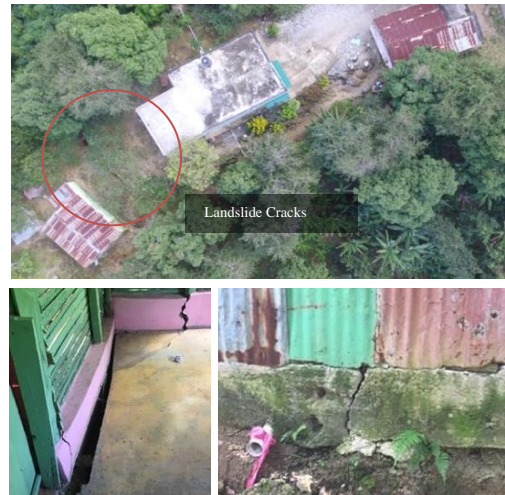
Figure 3. House foundation cracks
