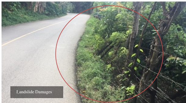
Figure 2. Highway affected by landslide
