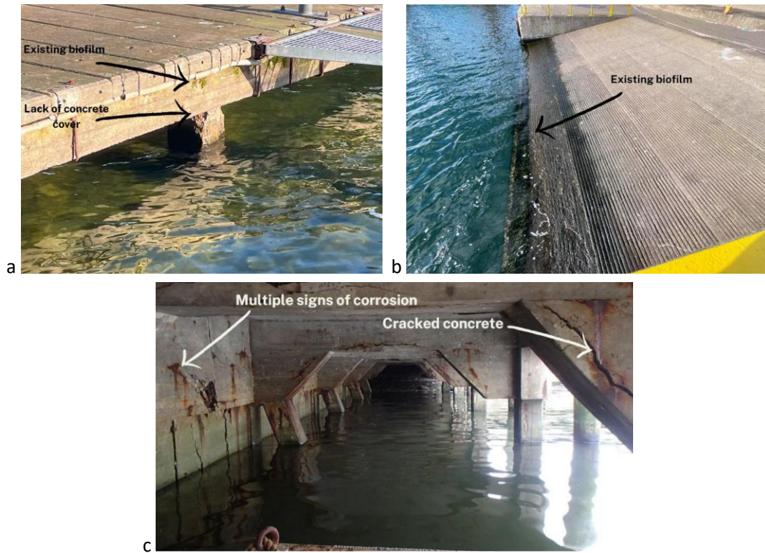
Fig. 1. Examples of damaged marine concrete structures – (a) Old Pier in Puck, Poland; (b) Seaport in Władysławowo, Poland; (c) Fur Harbour, Denmark.
