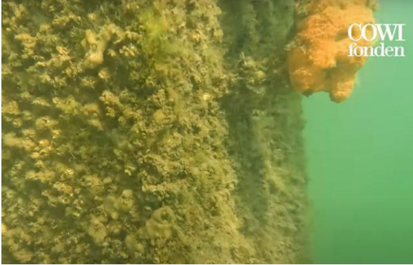
Fig. 4. Biofouling (growths and barnacles) visible on the surface of a submerged concrete pile.
