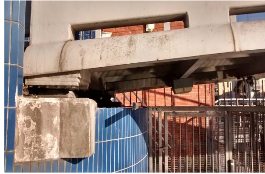
Figure 1: Photograph showing the location of the north-side bearings of Centenary Bridge, Leeds, UK.
