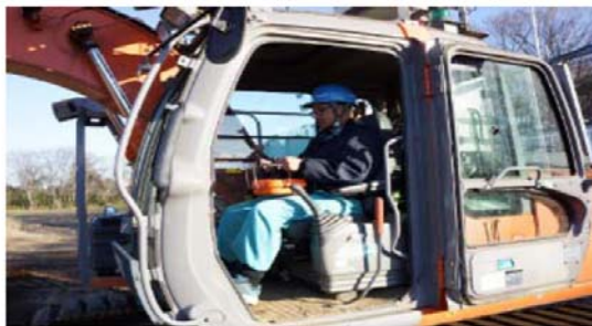
Fig. 3 Boarding operation using the remote control device
