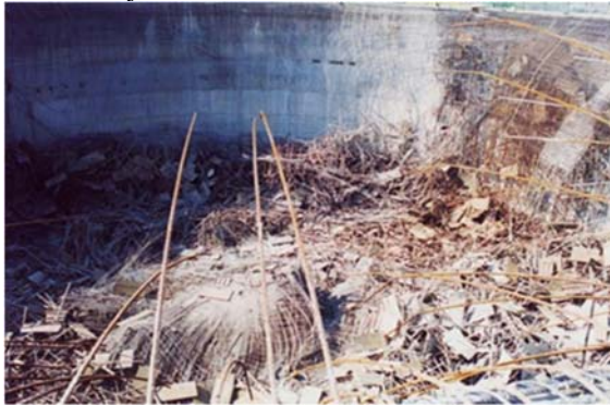
Figure 1. Formwork SSS collapse at the Beiling Boost Station Service Reservoir Project in Gangshan, Kaohsiung [5]
