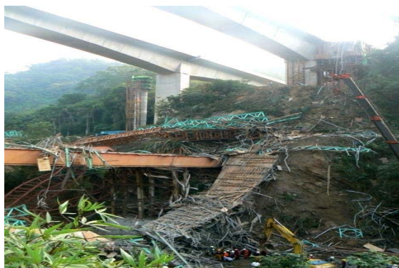
Figure 2. Formwork SSS collapse at the Beishan Interchange Bridge Project of Highway 6 in Nantou [6]
