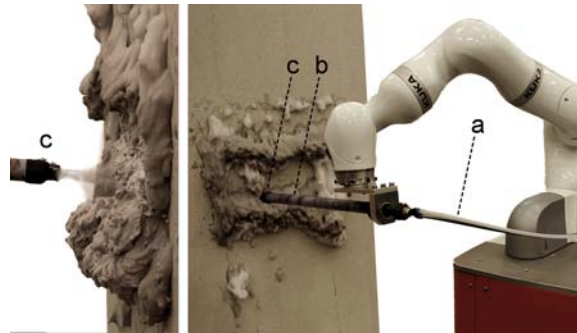
Figure 7. Semi-automated robotic foam concrete application with (a) separate material supply of foam concrete slurry and foaming agent (b) mixing of material components with modified foam branch pipe (c) conical tool tip
