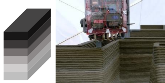
Fig. 6 left: Approach of CONPrint3D ® right: Extrusion of smaller concrete strands with round corners and subsequent concrete filling [8]
