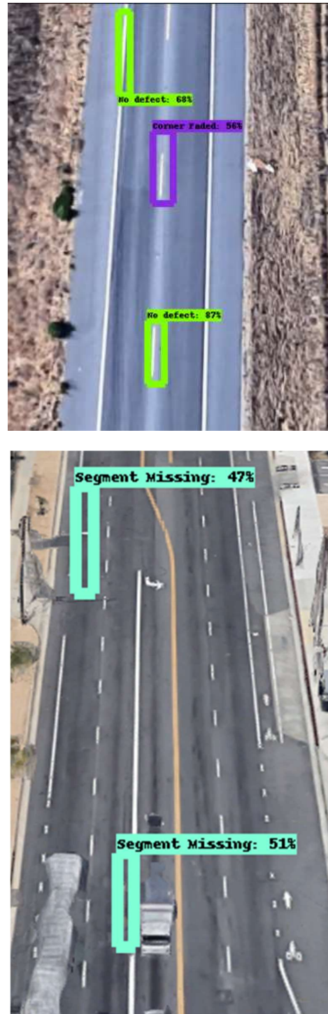
Figure 4. Defects Detection by the Deep Learning Model
