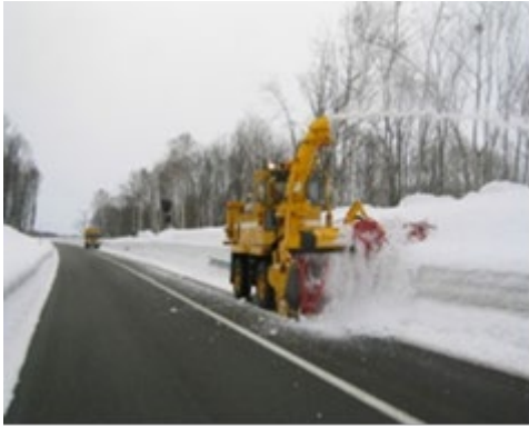
Figure-1. Snow and ice countermeasure work on the expressway (snow blowing work)
