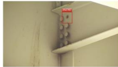
Figure 22. Defects detection from Drone bridge inspection
