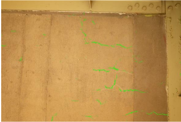
Figure 4. Bridge deck crack extraction image
