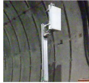
Figure 4. Portable 5G facility installed in the tunnel (4.85 Ghz, 120 W).
